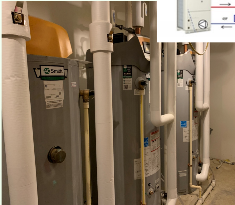
EMERALD HILLS APARTMENTS - CENTRAL CONDENSING GAS HEATERS
