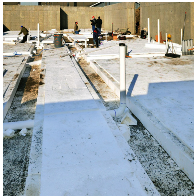
A thermal cushion for a building to sit on. Six inches of insulation is installed along with plumbing rough-in before the slab is poured for Sunshine Health Facilities' new administration building in Spokane, WA.
