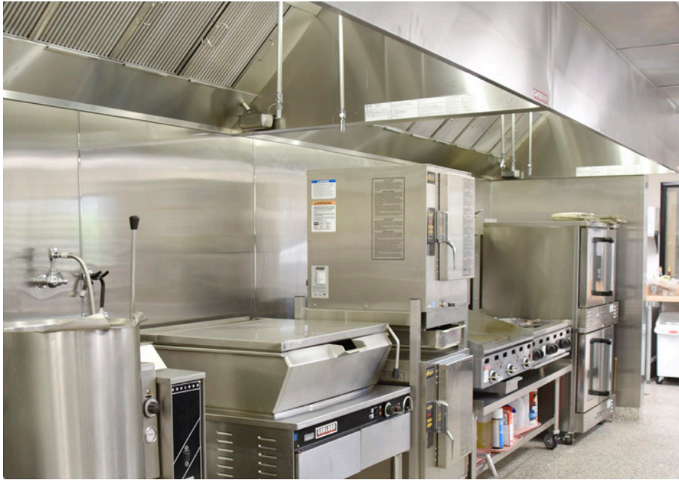
Commercial kitchens are afterburners for energy use. Grills, dishwashers, and ovens use a lot of power and create indoor pollution. Range hoods and dishwasher hoods quickly remove moisture and pollutants along with thousands of cubic feet of air. Dedicated makeup-air equipment is needed to balance this heavy exhaust. Photo taken at B on floor plan.
