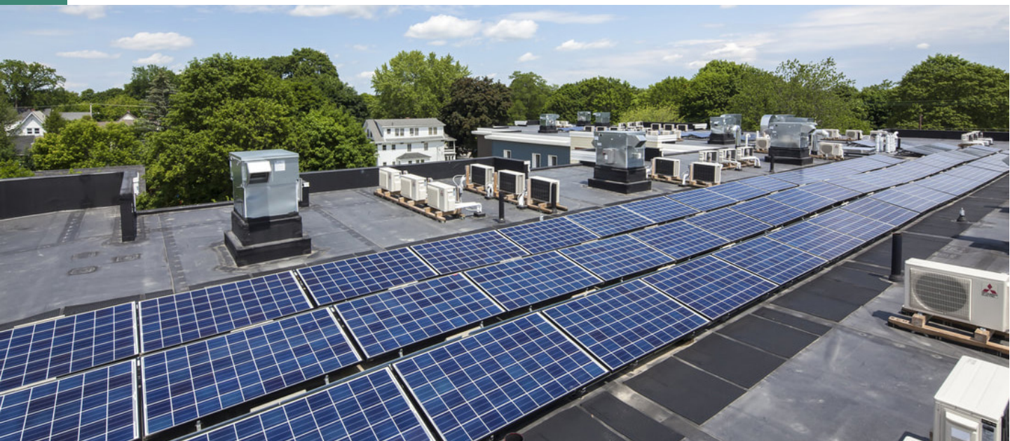
Energy misers and energy producers. Multiple minisplit heat pumps share the rooftop space with photovoltaic panels that provide 26 kW of free electricity—.
