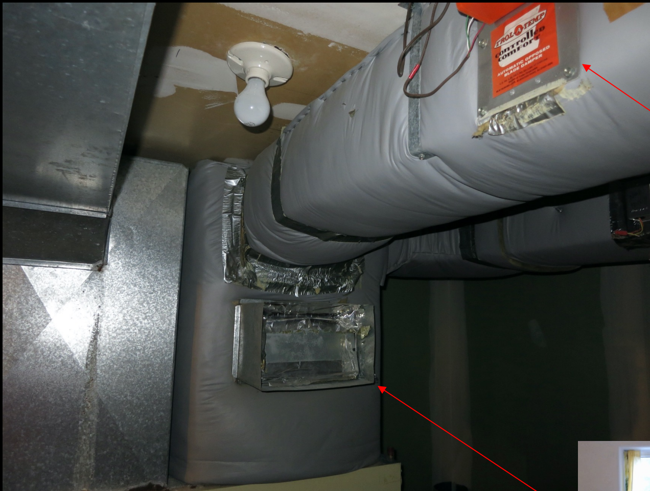
MOTORIZED ZONE DAMPER (1 OF 3)
