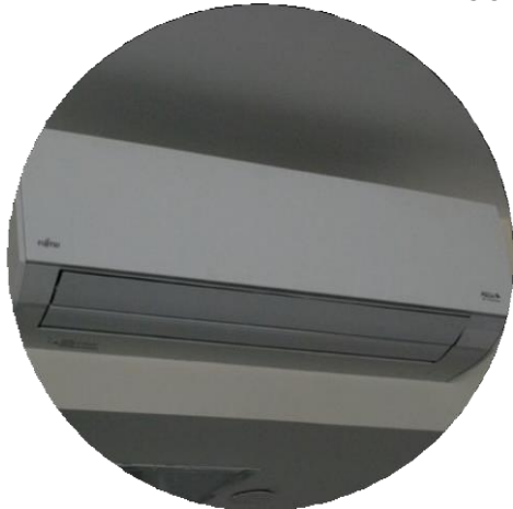
WALL MOUNTED HEAT PUMPS IN 1 BEDROOM UNITS
