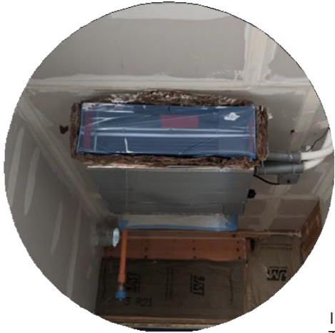
DUCTED HEAT PUMPS IN 2 & 3 BEDROOM UNITS
