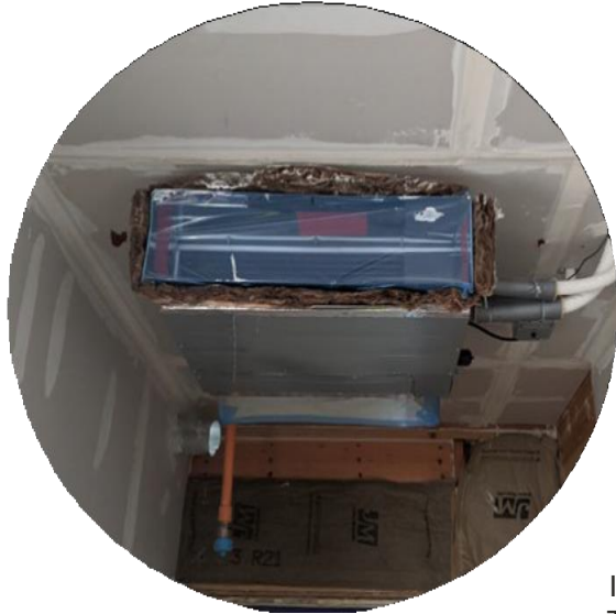
DUCTED HEAT PUMPS IN 2 & 3 BEDROOM UNITS
