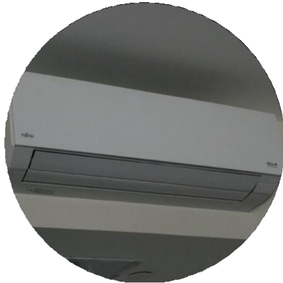
WALL MOUNTED HEAT PUMPS IN 1 BEDROOM UNITS
