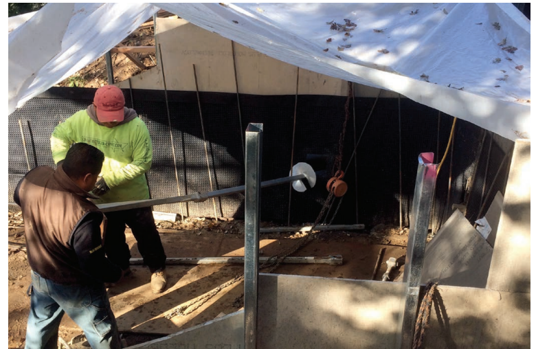
A Shotcrete Retaining Wall Shoring up an unstable slope, with minimal formwork
