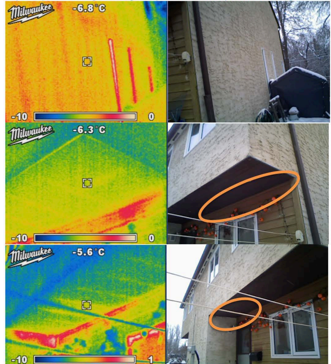
Figure 9: Infrared Thermal Images of Sundance Unit #15, taken just after sunrise on November 15, 2017. IR images shown on the left, with corresponding regular image shown to the right. The color legend represents the range in temperature present in the image; note that glass temperature is not accurately reflected in these images.
