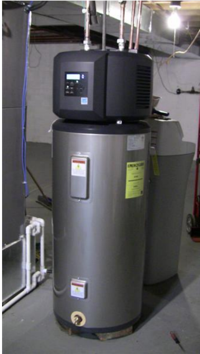
Heat Pump Water Heater
