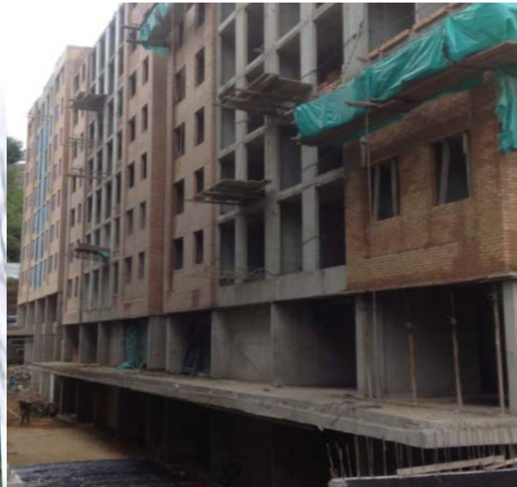
Requires a Transition Slab for Underground Garage
