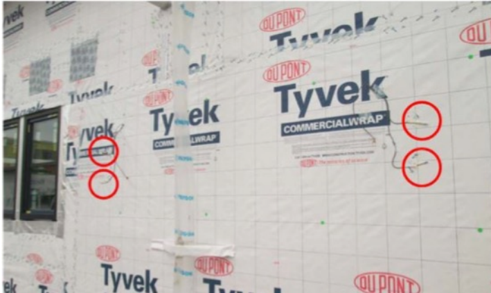
1. RH/T sensors on exterior drainage plane
