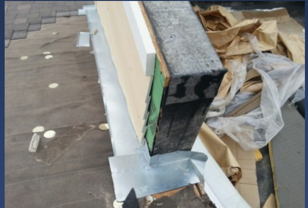
No Strip-in Flashing
