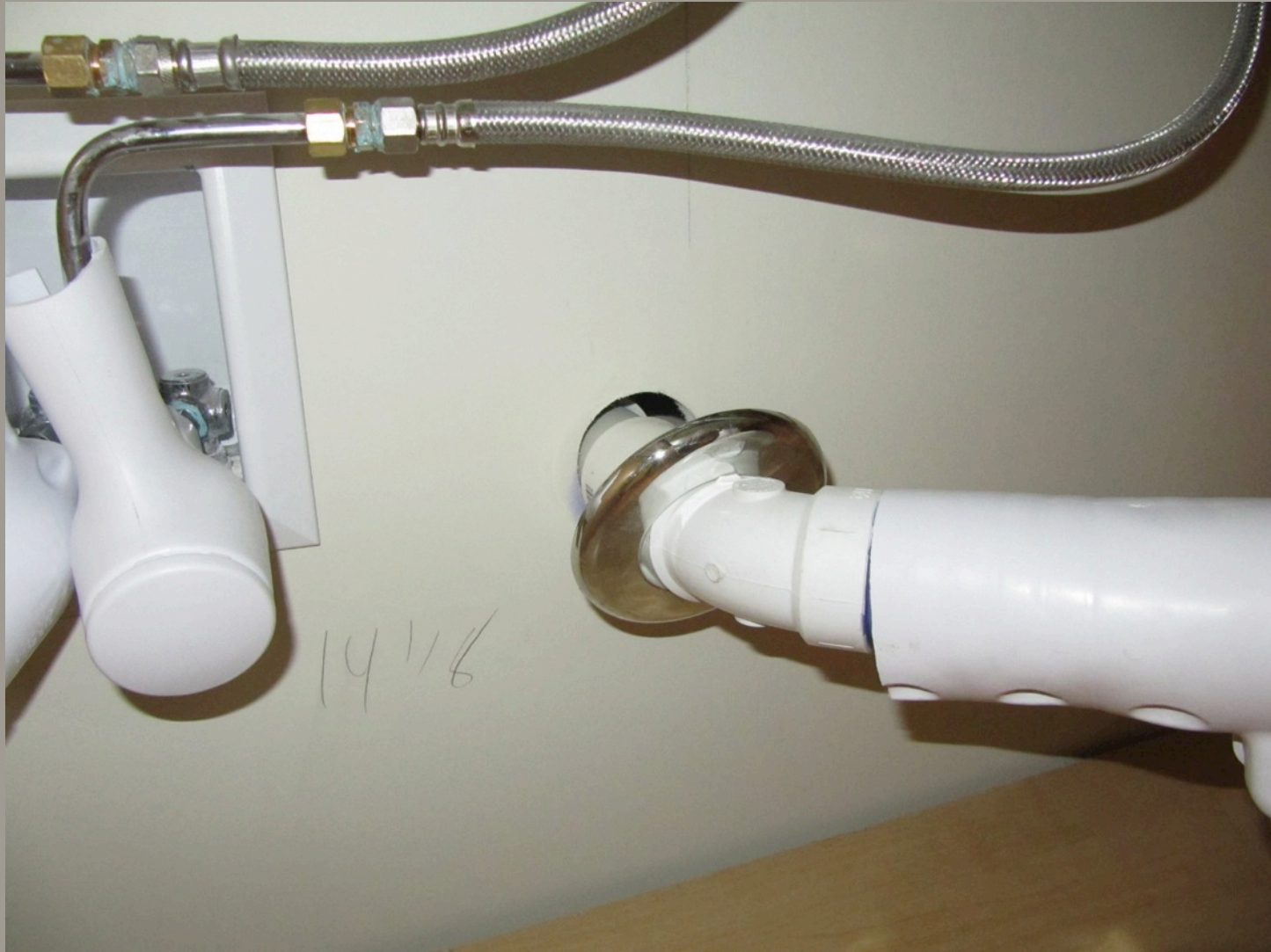
Hunting for Air Leakage
