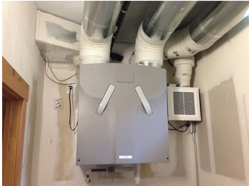
HRV w/bypass; Exhaust fan to laundry room
