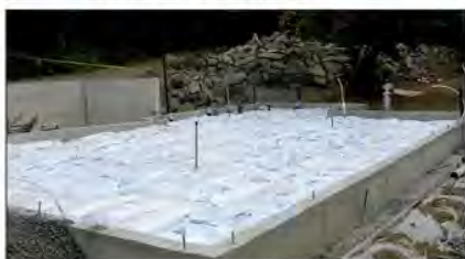
Top: placing unopened perlite bags on grade. Above: perlite bags packed tightly in place.
