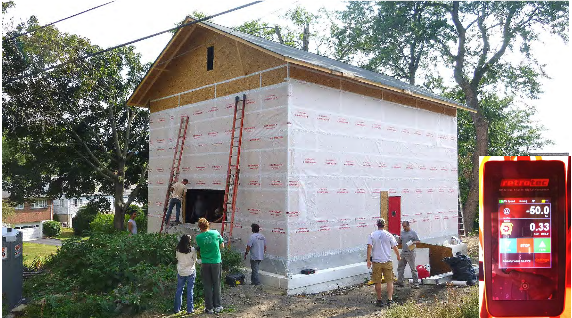
Richard Pedranti, architect and Pete Vargo, PHIUS+ energy rater performing initial blower door test
