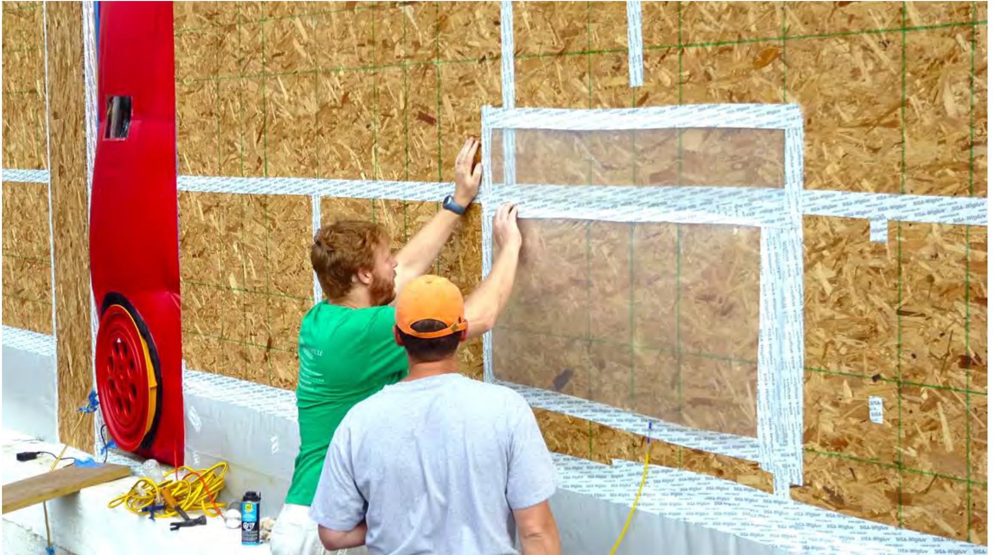
Owner, Declan Mulhall and PHIUS + rater, Pete Vargo during balloon test #2 over OSB panel only
