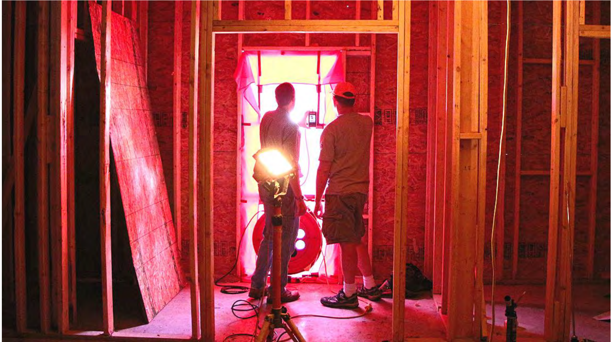
Richard Pedranti, architect and Pete Vargo, PHIUS+ energy rater performing initial blower door test
