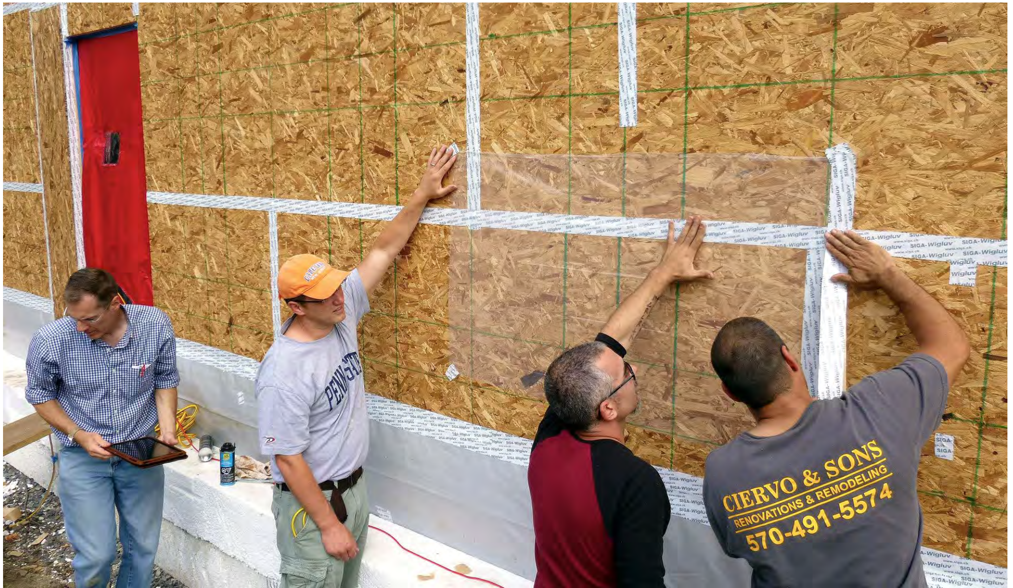
Preparing positive pressure balloon test #1 on OSB panel and seam taped with SIGA wigluv
