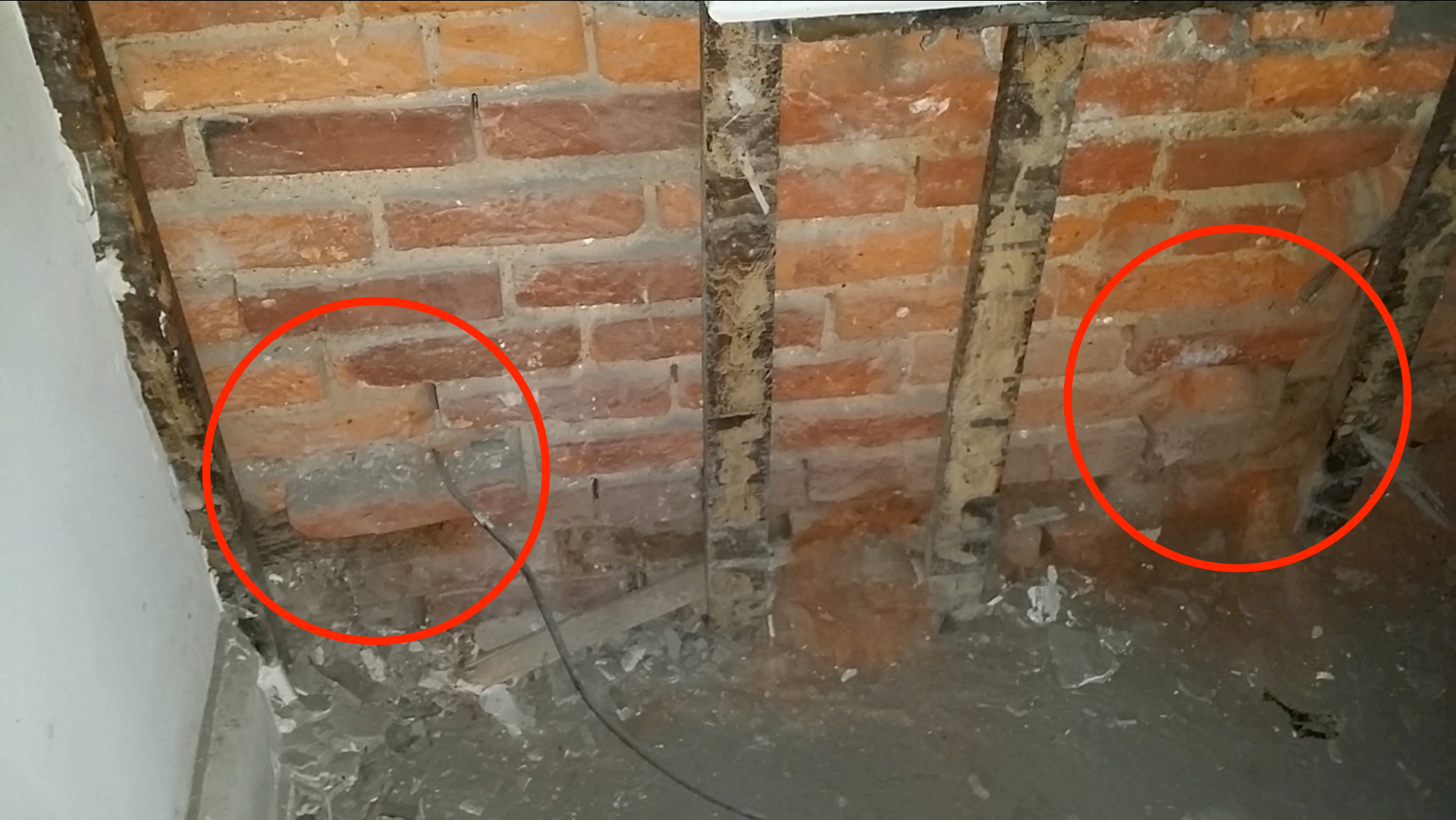
Deteriorating Brick Walls
