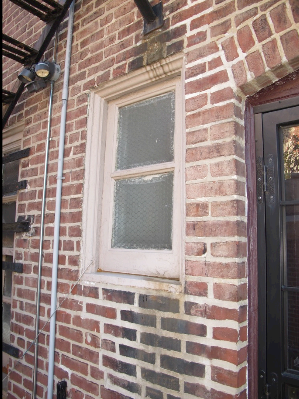
Deteriorating Brick Walls
