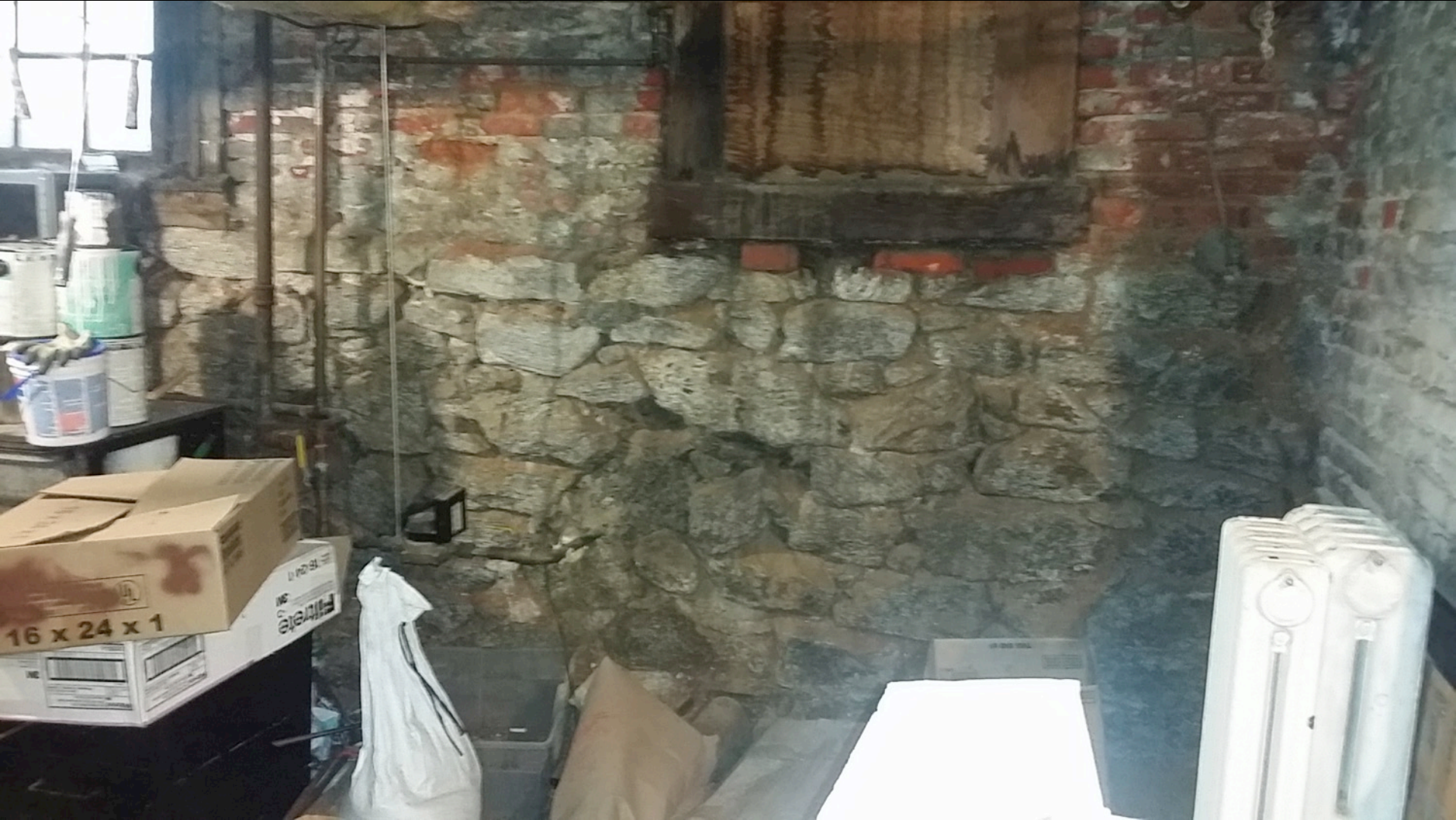
Deteriorating Stone Walls
