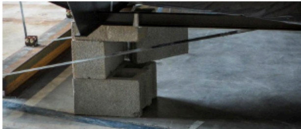
Figure 2.3. Ineligible dry-stack foundation
