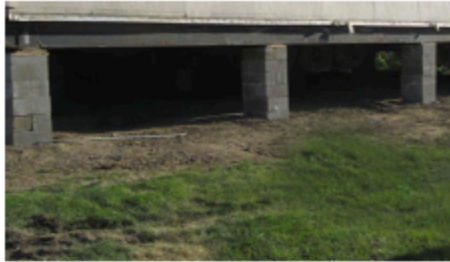
Figure 2.1. Ineligible dry-stack foundation
