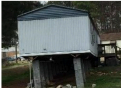
Figure 2.2. Ineligible dry-stack foundation
