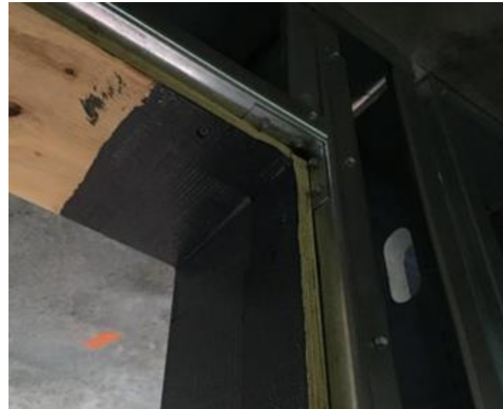
Liquid flashing at upper corner of window
