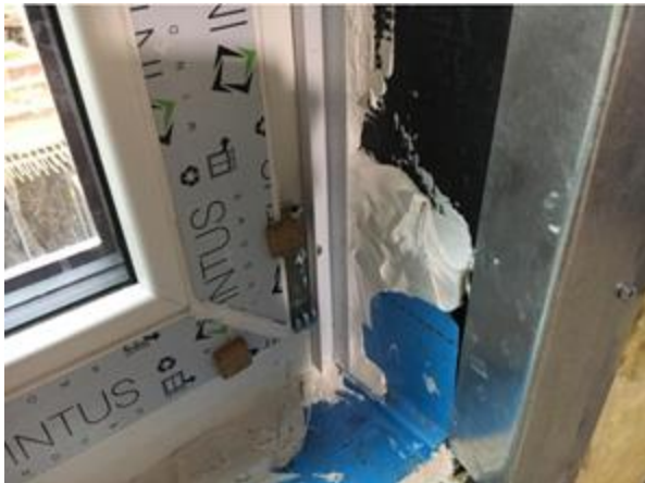
Liquid flashing at upper corner of window
