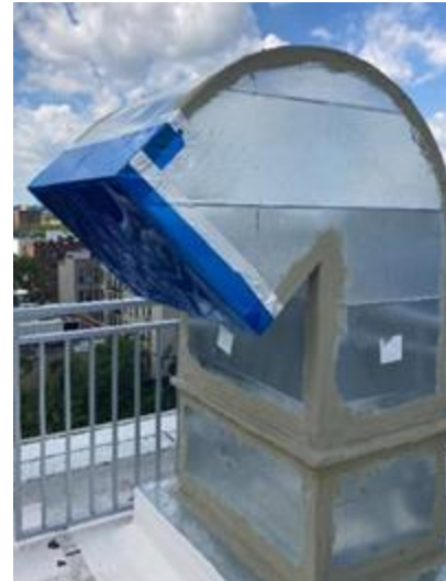
Dryer exhaust temp. seal
