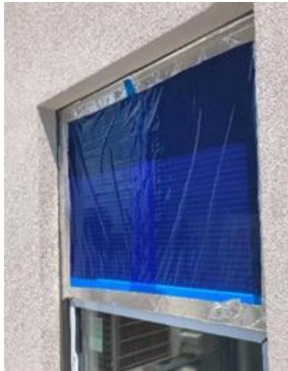
Smoke vent louver temp. seal
