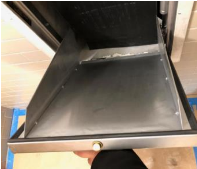
Trash chute gasket
