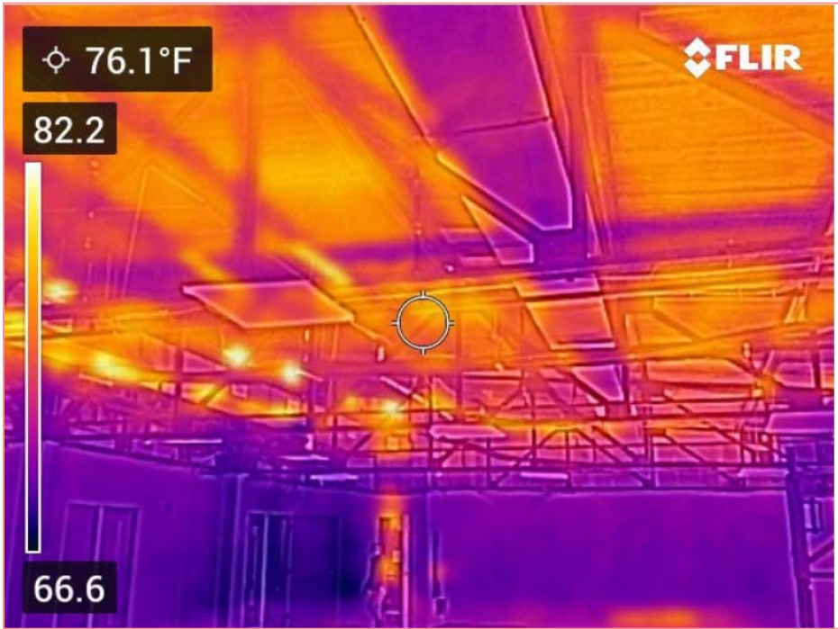
BSC Report: pg 37, Figure 111 Roof 2 nd floor east. Extreme heat transfer due to very poor thermal performance. This results from solar gain of roof. Outside temperature at the time of reading was 65F.
