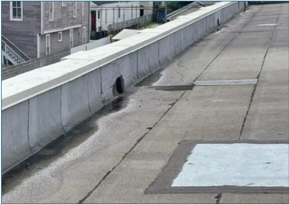
KL site images Standing water on roof at east parapet wall may be related to areas of high moisture content and may be related to wet batts noted in BSC Report: pg 18, Figure 40
