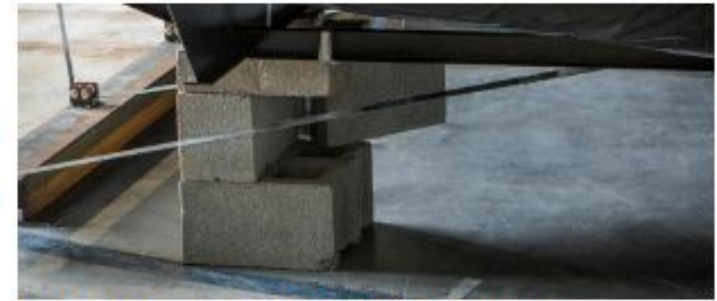
Figure 2.3. Ineligible dry-stack foundation
